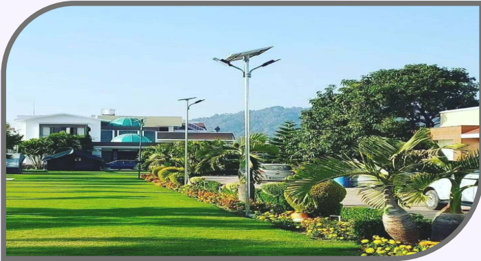
Himurja (Himachal Govt. Project) 50k+ Successfully Installed
